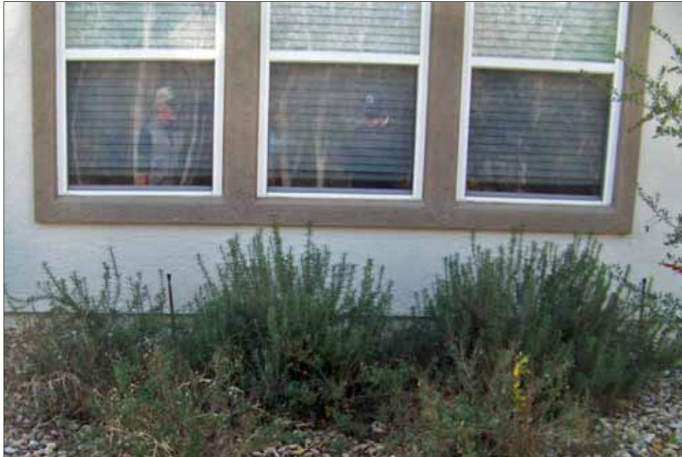
Rosemary needs to be at least 3 feet from the foundation.
